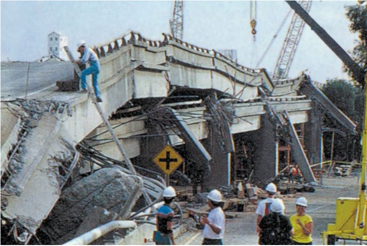
Figure 12.14 A collapsed section of the Cypress Freeway in Oakland California. Source: U. S. Geological Survey (1989) Public Domain view source
