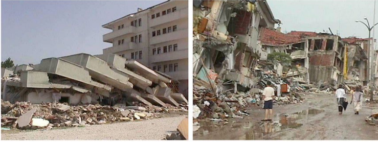
Figure 12.15 Damage from the 1999 M7.6 Izmit, Turkey earthquake. Source: Left; USGS (1999) Public Domain view source; Right: USGS (1999) Public Domain view source
